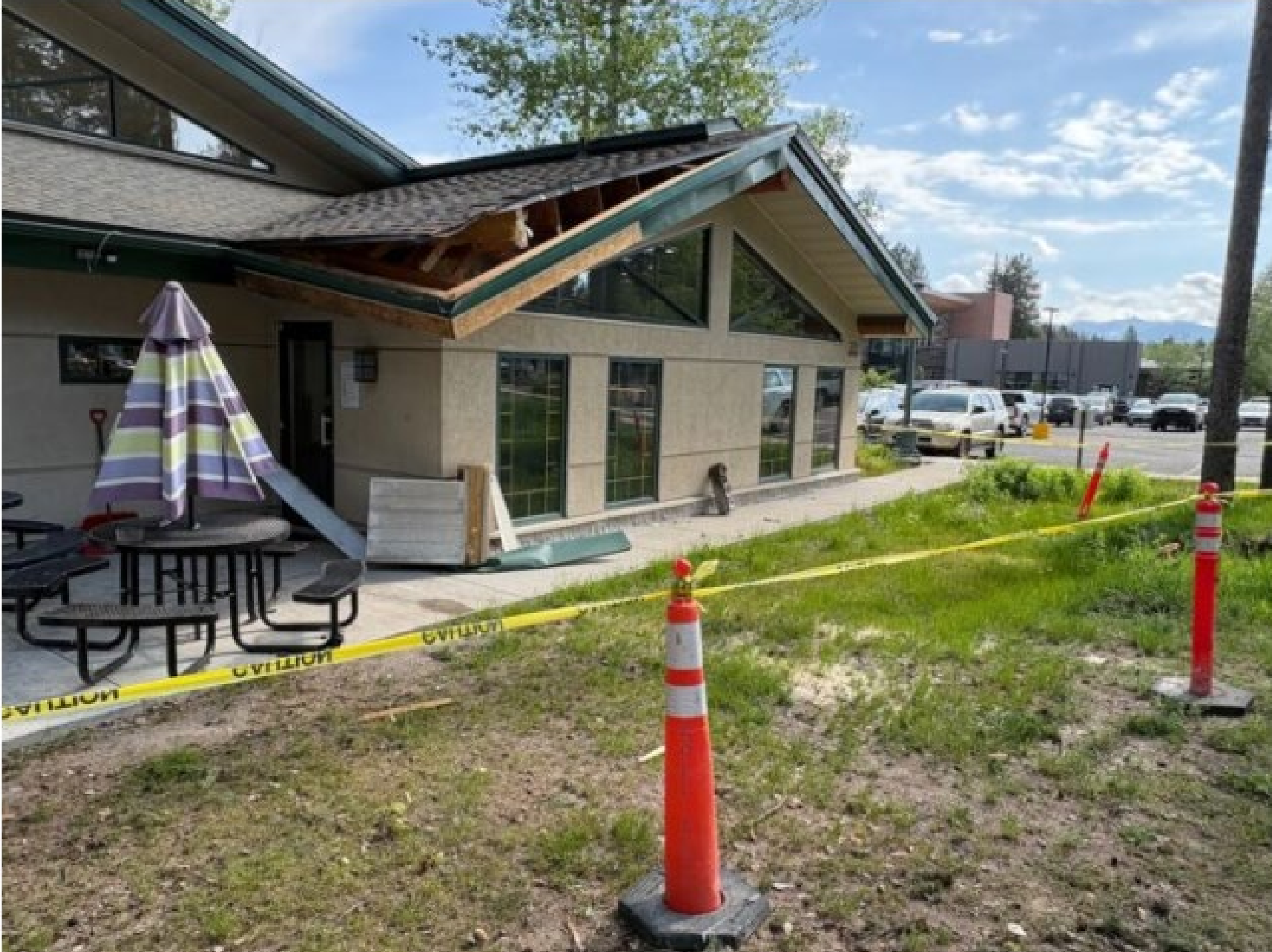
Damage to the roof of the Payette Lakes Medical Clinic. Photo: Drew Dodson/Valley Lookout
