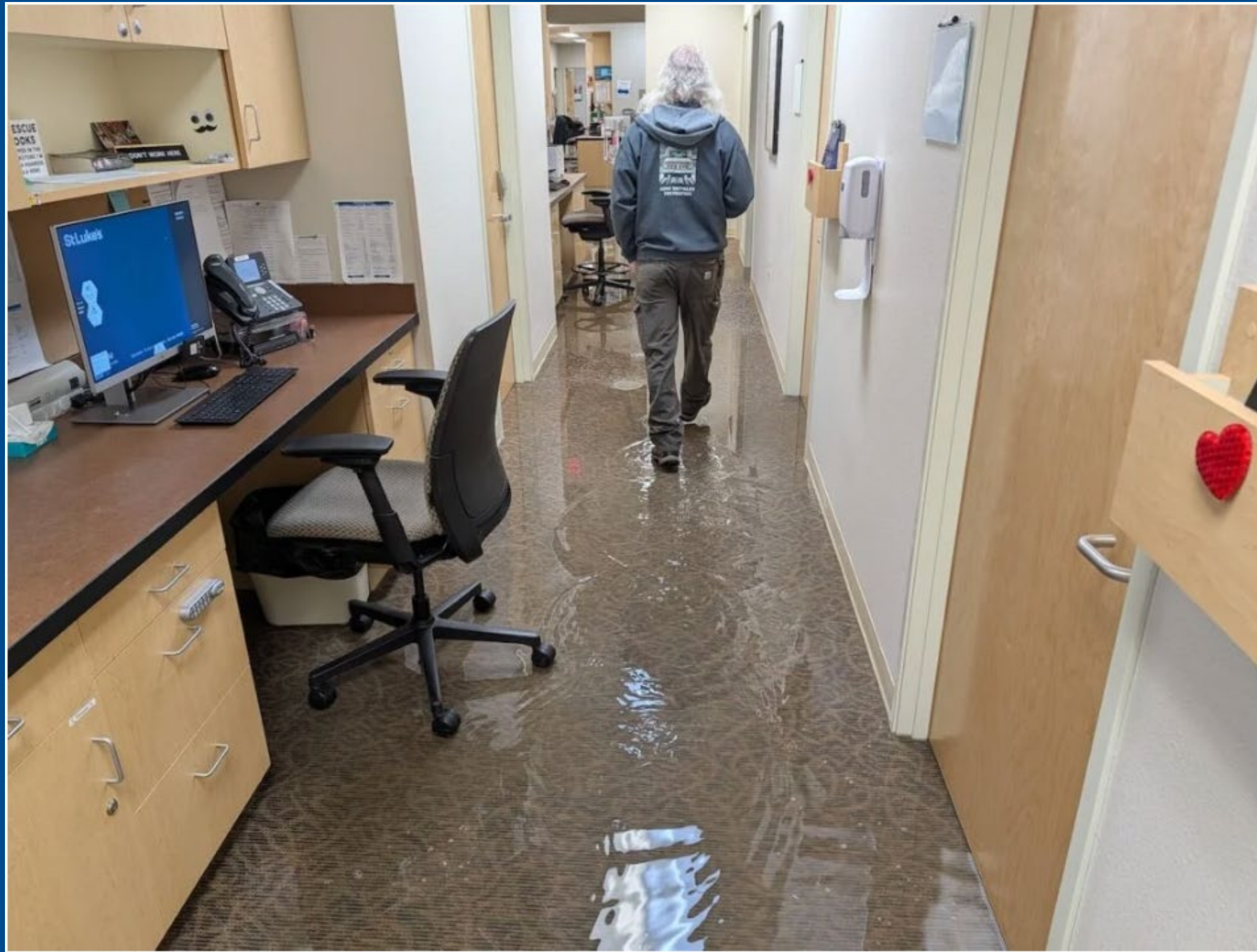
Levi Brinkley of St. Luke's McCall Building Services team assesses the water damage at St. Luke's McCall Medical Clinic. Photo: Courtesy St. Luke's McCall
